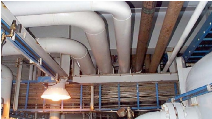
RACKING UP THE YEARS I-Rod was used to dress beams beneath multiple pipes. No corrosion at 13 years.
