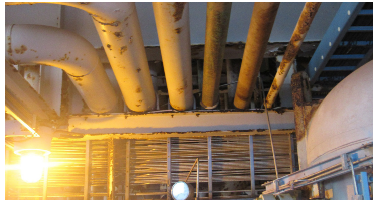
HOLDING UP WELL I-Rod supporting multiple pipes across a standard beam support.
