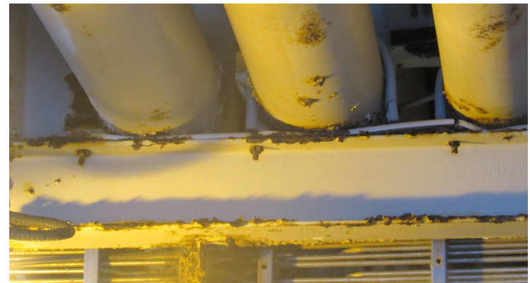
VERY LITTLE CHANGE 15 years later, the crack has not compromised the support or intensified corrosion.
