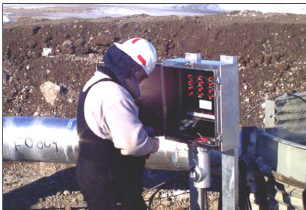
Outdoor panel on pipeline system in Alaska
