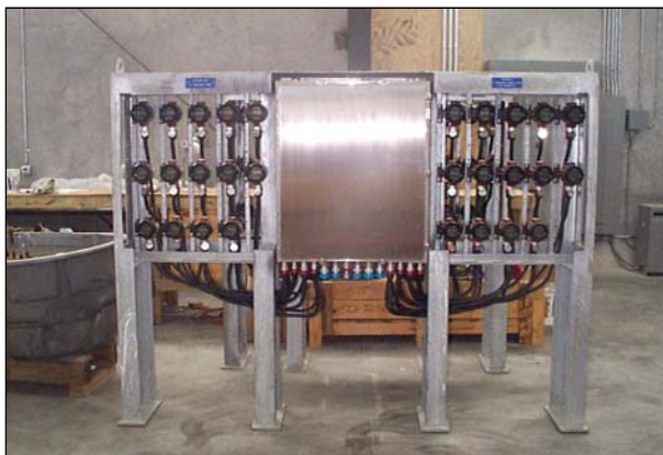
30 channel SCADA linked panel
