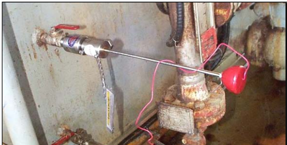
The Polatrak RT-1Z in situ.
