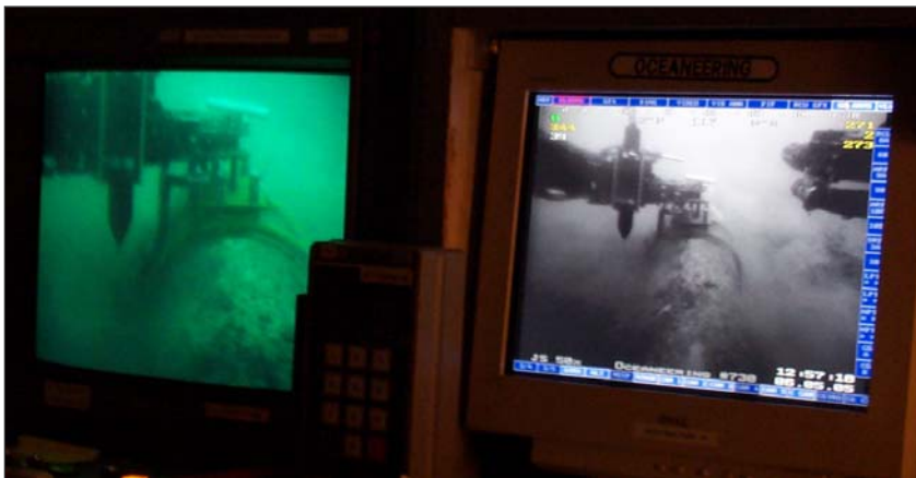
An ROV installation of an ExpandaSled™ and RetroClamp. Pipelines only have to be partially excavated.
